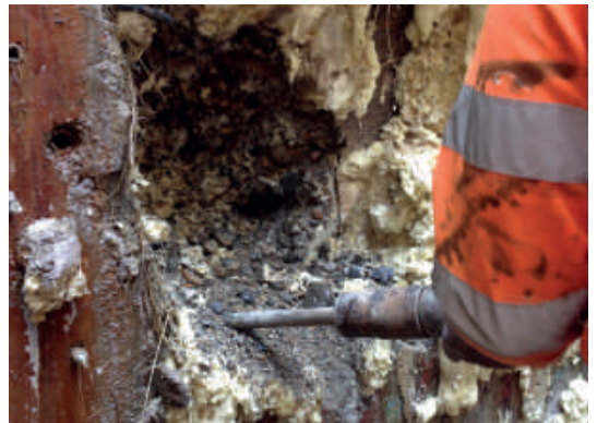
Breaking out for opening of a heading to connect to a pipeopening
